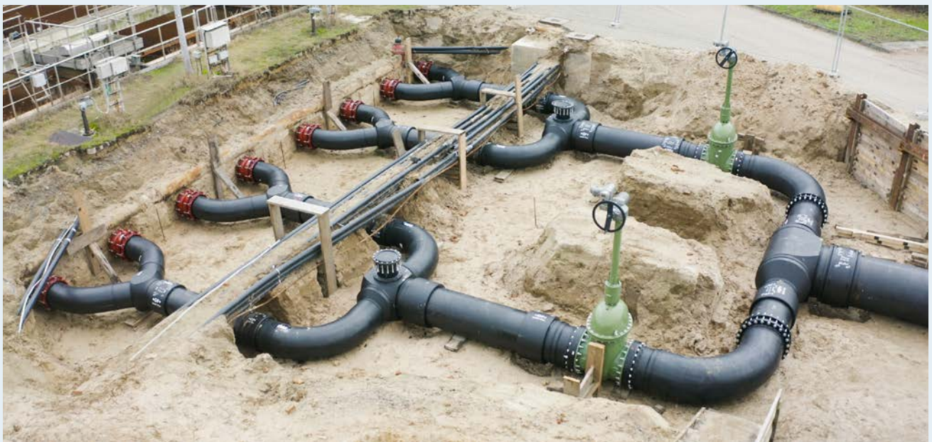
One of three cascades being replaced with flow solutions from GF during ongoing operations at Berlin's largest wastewater treatment plant.
